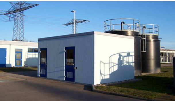
Station zur Phosphatelimination
